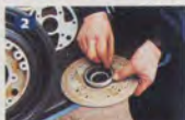
2 New 'O' ring being placed on to the top of the clamp plate.
