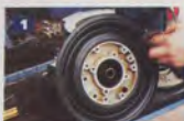
1 New seal in place on gear box. Don't use any sealing compound.
